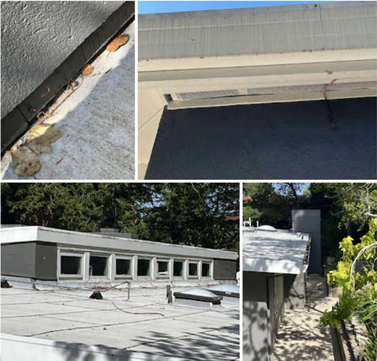
Photos (clockwise from upper left): 6" combustible siding below stucco base, gap in soffit screen, clerestory windows, debris in gutters.
