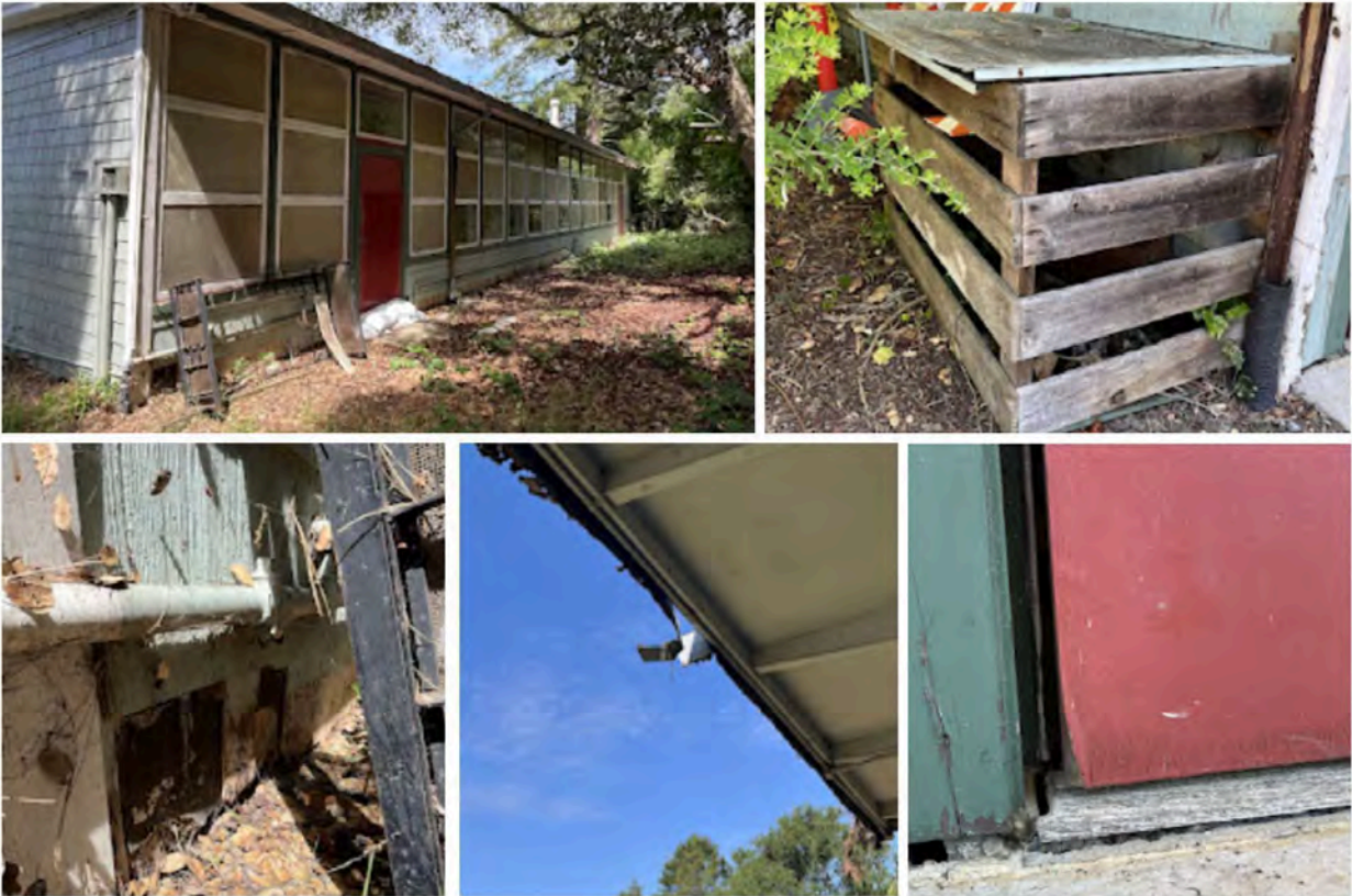
Photos: View of building from rear showing worn siding, missing windows, and multiple areas of decay.
