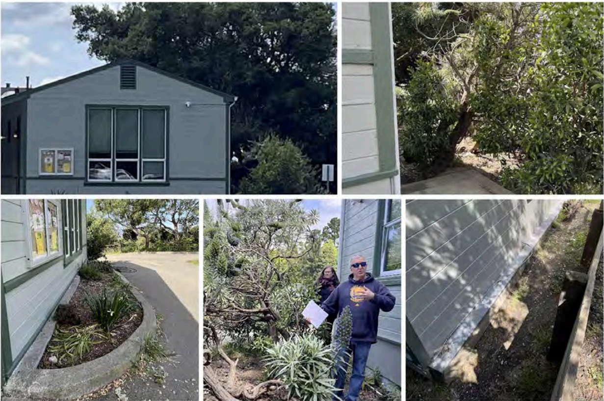
Photos (clockwise from upper left): view of trees and vegetation overhanging structure; vegetation in Zone 0 on NW corner; planter under north-side windows; overgrown vegetation on NW corner; wooden retaining wall in southeast corner prone to collecting debris.
