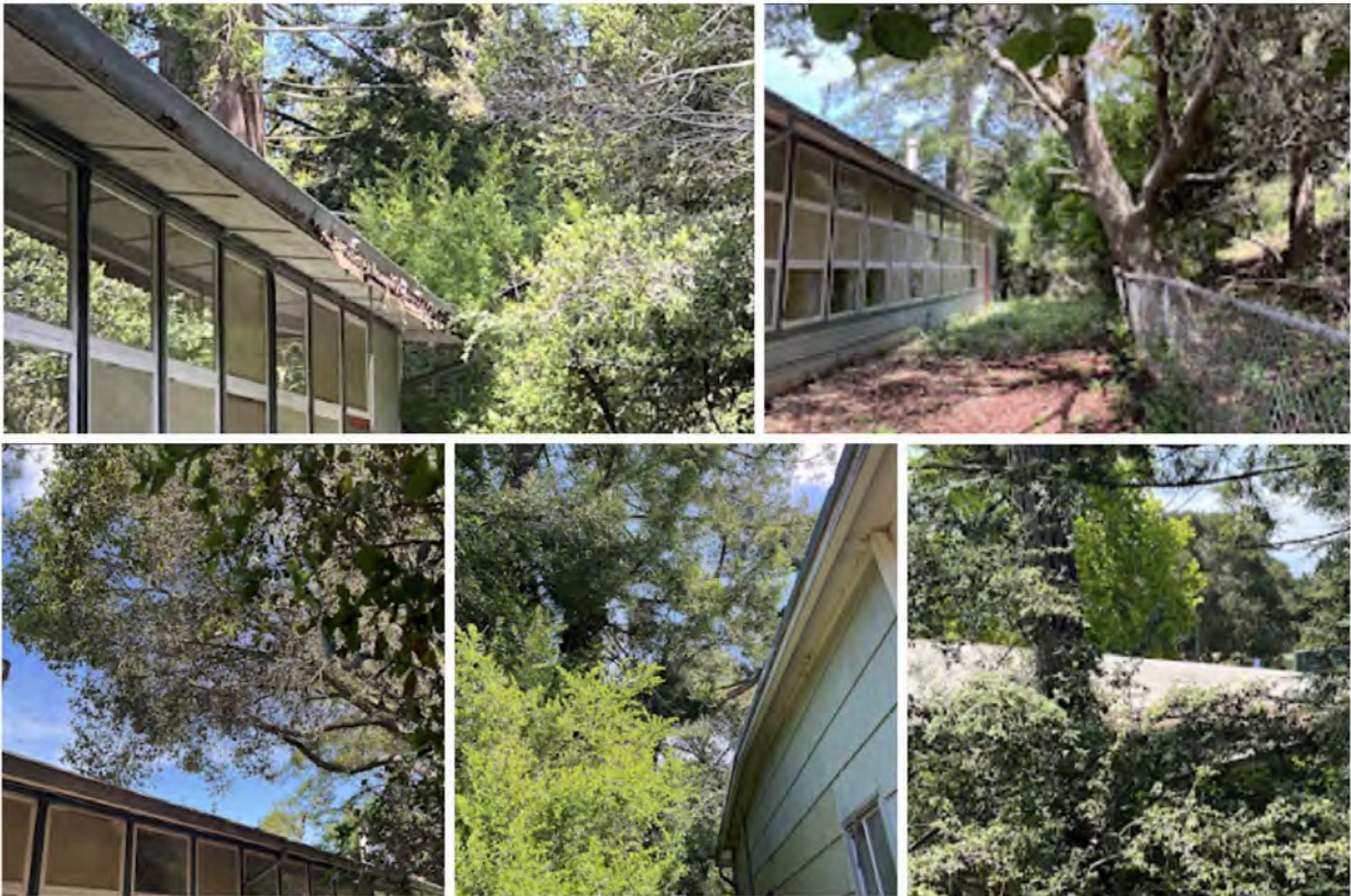
Photos: Views of dense vegetation between rear of building and Kensington Park Road, ladder fuels, and tree limbs overhanging the building.
