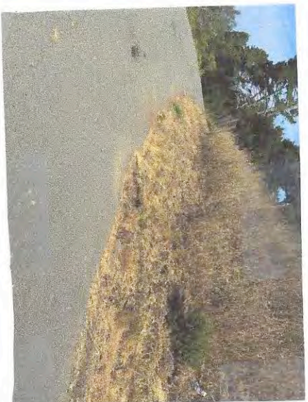
Turn in road, needs hillside barrier
