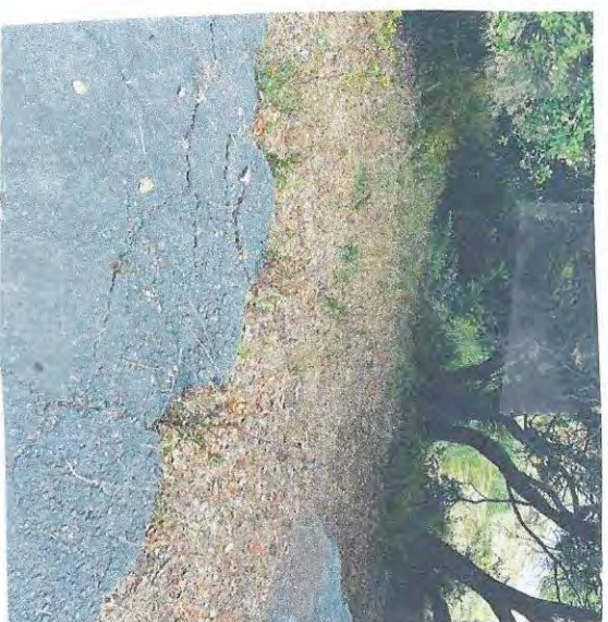
Erosion on south hillside needs water barrier
