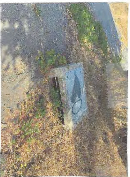
Catch basin for road water needs cleaning & hill barrier
