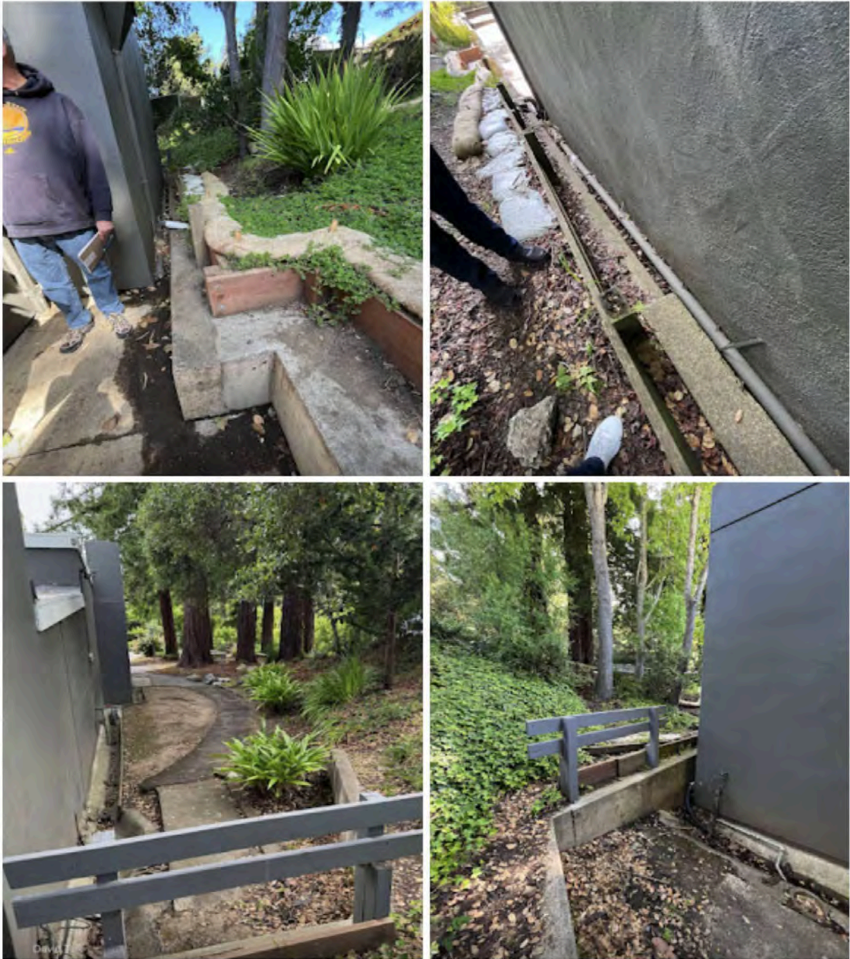
Photos (clockwise from upper left): Water management system and wooden retaining wall traps debris on the east side.
