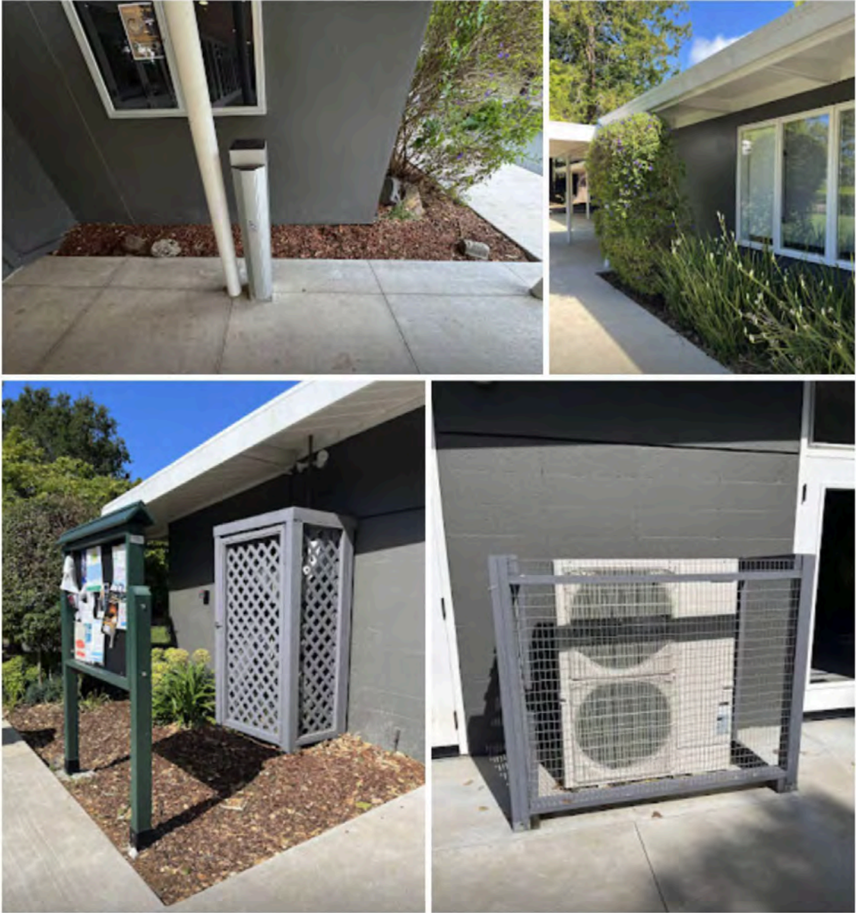
Photos (clockwise from upper left): L-shaped planter with mulch and vegetation beneath eaves at front; wooden screens for mechanical equipment on side.
