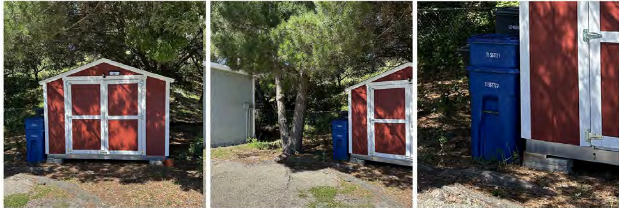
Photos(from left): View of new shed, proximity to annex and tree with overhanging branches; and combustibles, debris and open base under the structure.
